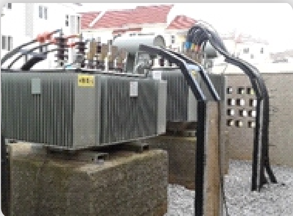
1.0MVA 0.415kV/33kV Substation
