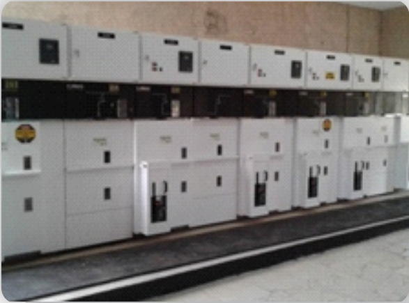
33kV Switchgear Panels at Brains & Hammers
