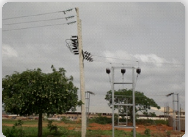
33/11kV Substation Yard
