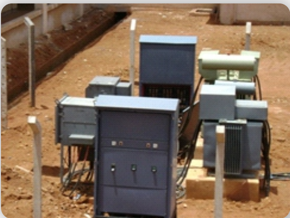
11kV/415V Substation Yard
