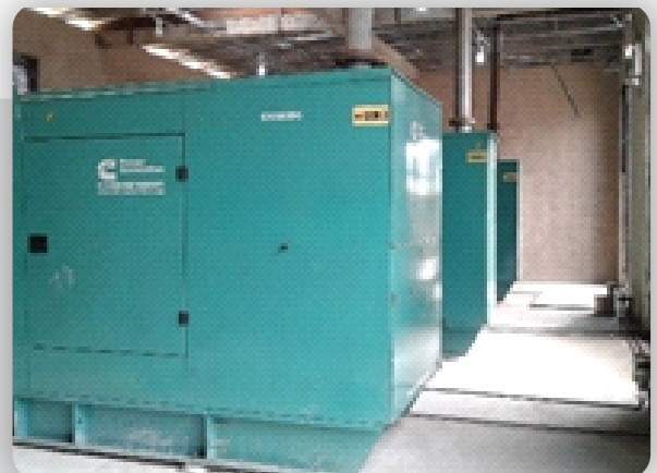
3x500kVA Genset at Brains & Hammer Life Camp
