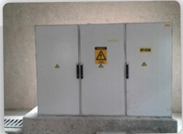
2500A Synchronizing Panel
