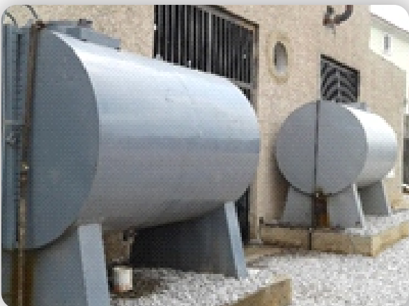
Diesel Day Tanks at Brains & Hammers
